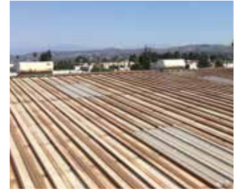
Rusted metal roof
